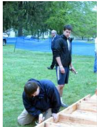
Julius Feniola & Ryan Monico, helping to Raise the Roof (Habitat) in Madison
