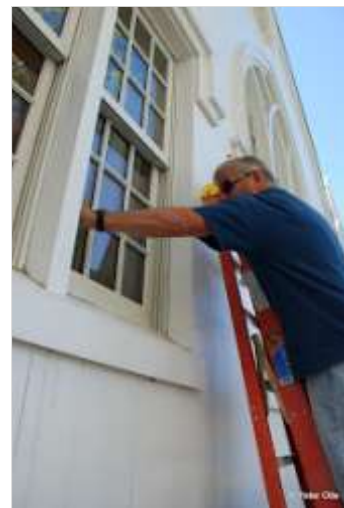
Work Day was a perfect spring day to wash windows, clean up the landscape, and more. Many thanks to the willing hands!
